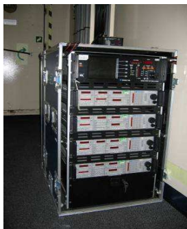
Figure 25. Telemetry receivers and signal combiner installed used by the test centre
