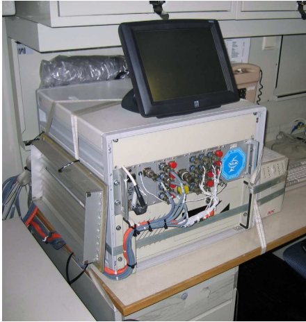
Figure 8. Data Acquisition Unit (DAU), installed in the vicinity of the wheel house
