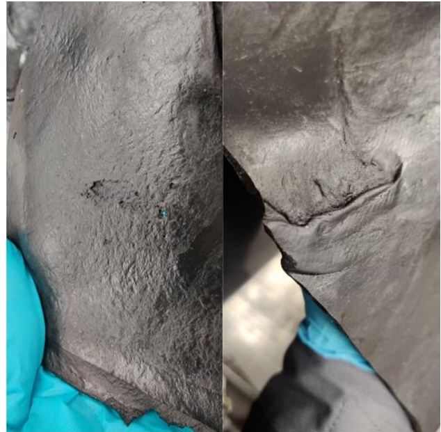
Figure 4: EPDM with pore (left) and material warpage (right)
