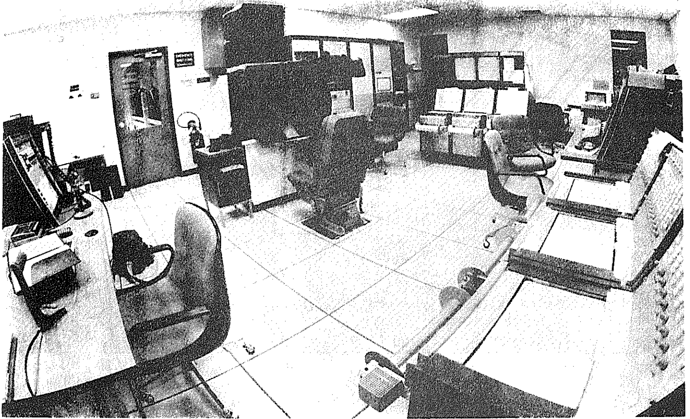
Fig. 8 VMS control room and red pilot station.
