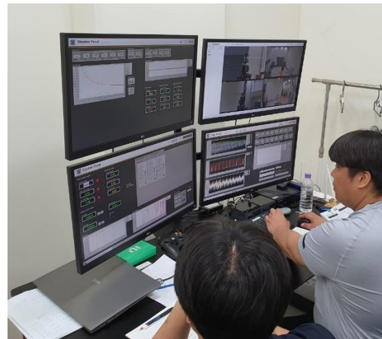
(b) SNURTS console monitoring room
