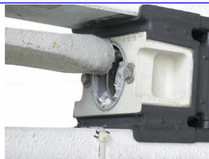
Figure 14: DAUPHIN tip arm failure
