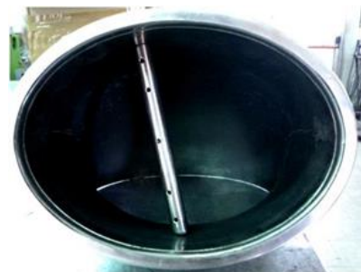
Figure 11. The sampling probe welded on the stack
