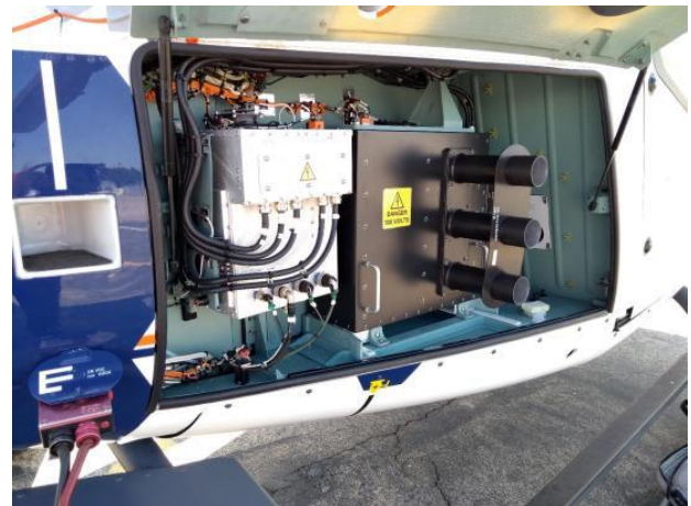
Figure 8 : View of the Inverter and the High Voltage Battery in the Right-Hand Cargo Bay of H130 Flightlab
