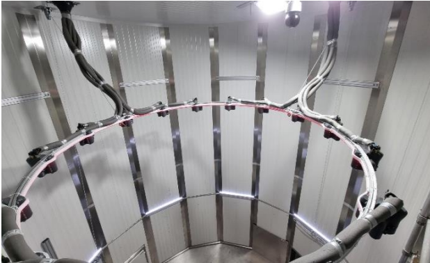
Figure 7: Installed spray ring system below the cooling chamber ceiling
