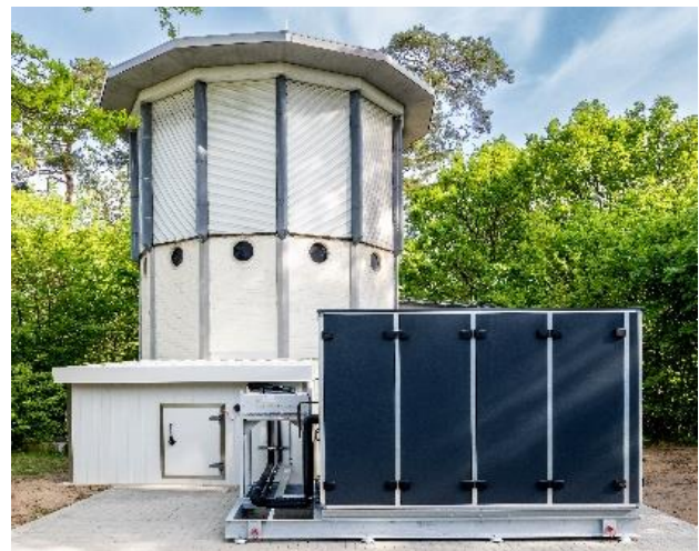
Figure 12: Components of the cooling system
